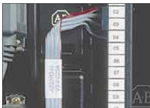
Terminal Block Labeling
